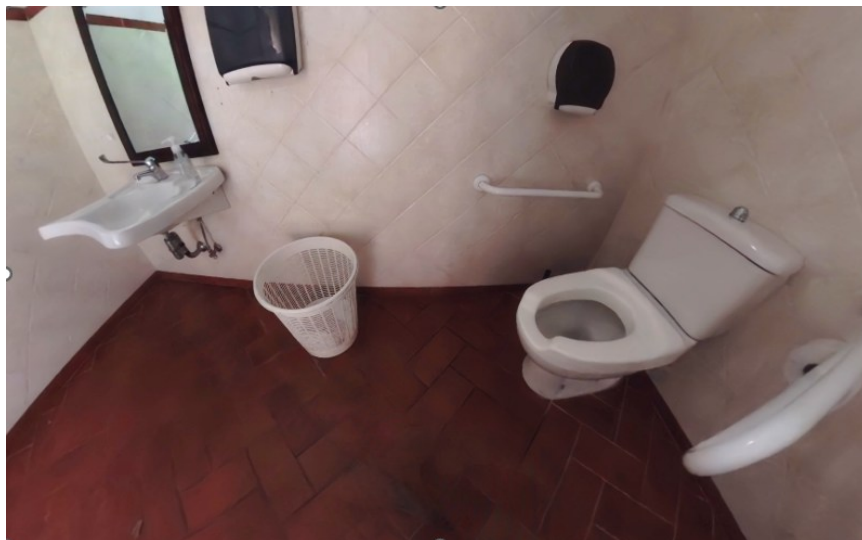
44 Bathroom interior Via Soccorso parking
